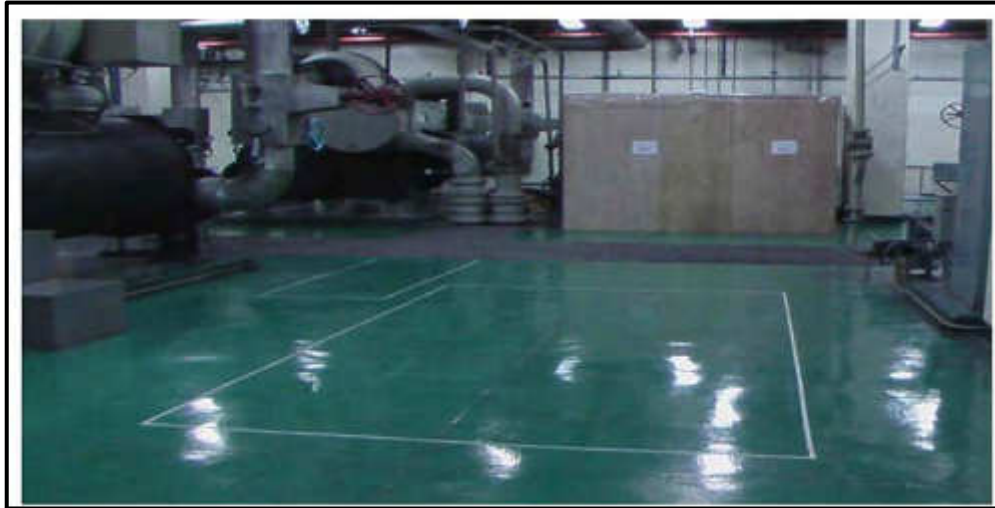
Photograph A3.2: Chillers
