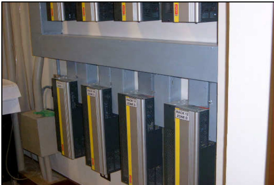
Photograph A4.2: New Dimmer Panels Racks
