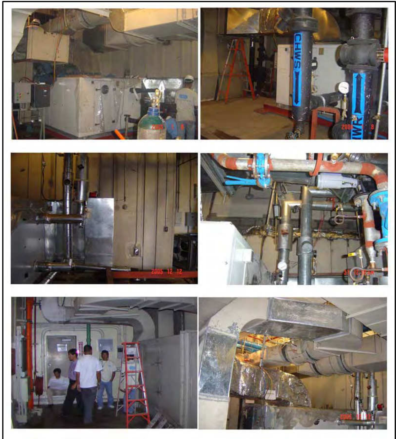
Photograph A3.1: Secondary Air Handling Units
