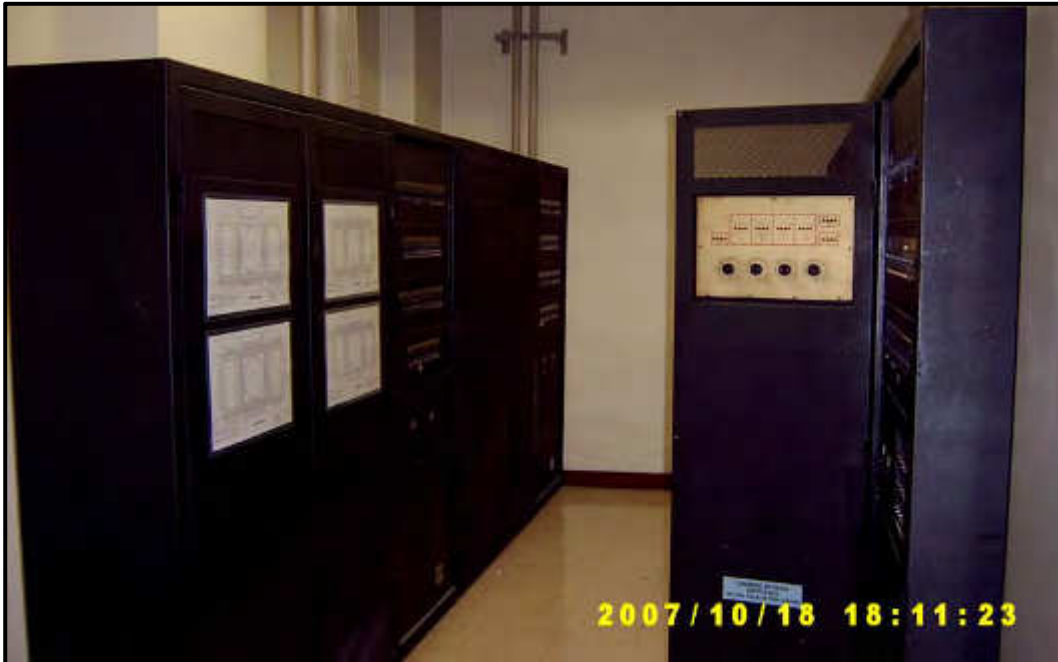
Photograph A4.1: Old Dimmer System Panel
