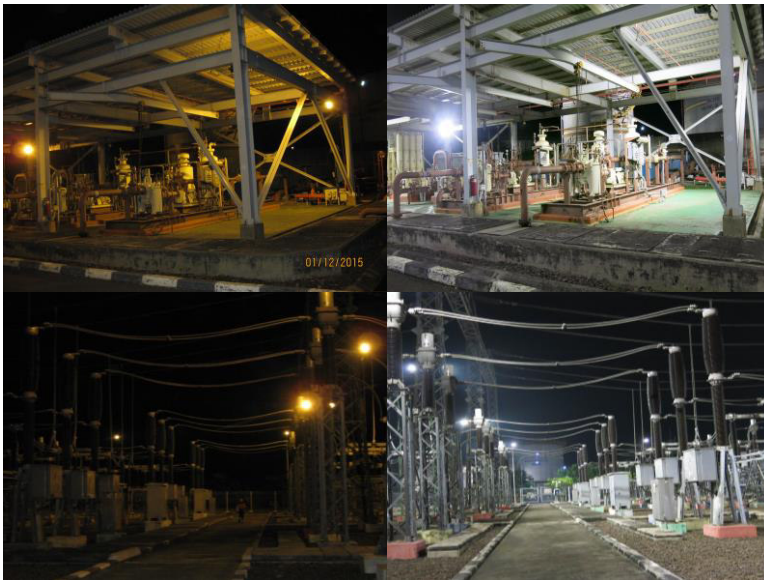
The retrofitted LEDs at the Cilegon Substation provided improvement in the uniformity ratio, bringing more evenly-distributed light, with lower wattage consumption.
