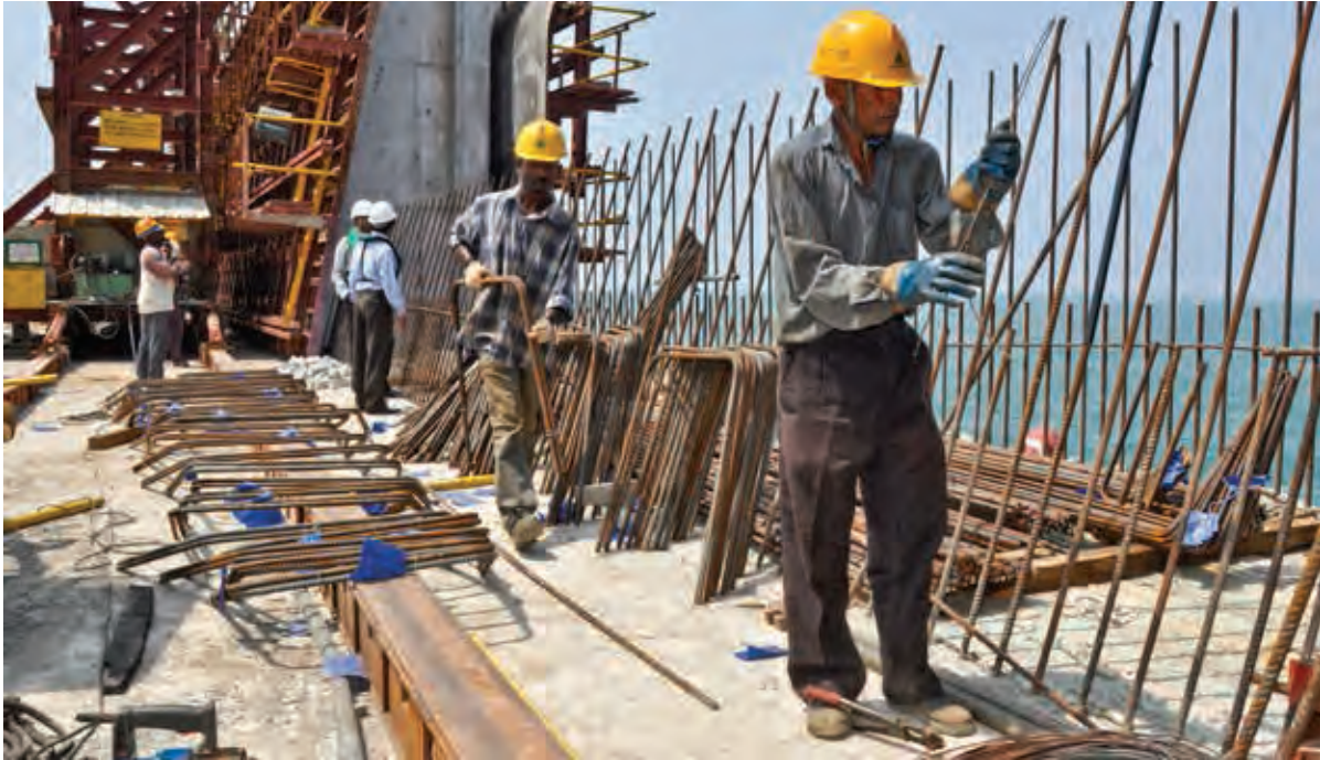
Construction works at the Colombo Port Expansion Project. James Hutchison | ADB Photo Library.
