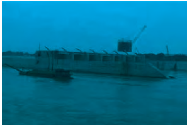
The shiplock under construction on the bank of the river. Source: ADB Photo Library.
