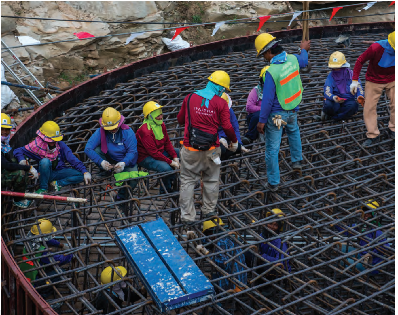
Construction for the foundation for one of the wind turbines. The tower will reach 120 meters, when completed.
