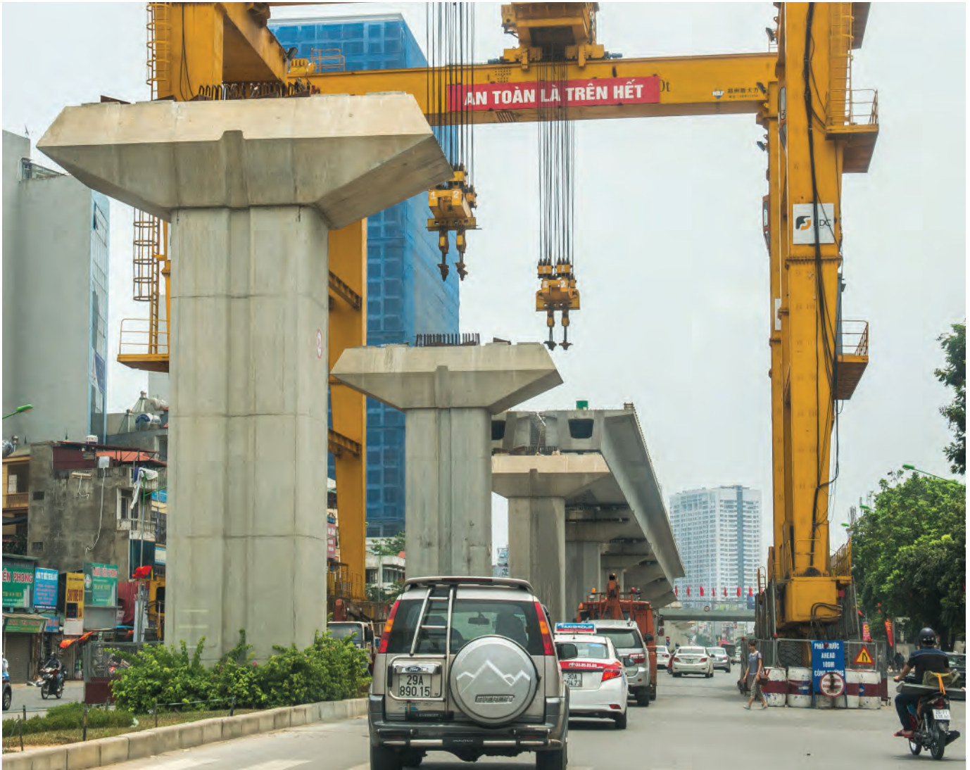
The Ha Noi Metro Rail System under construction. The metro Rail system is expected to ease traffic congestion and reduce emissions in Ha Noi.
