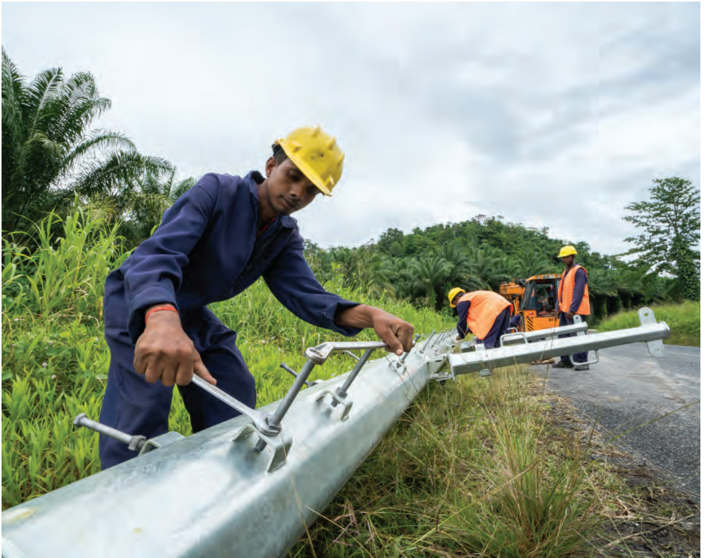
Workers installing transmission lines in Kimbe, West New Britain, Papua New Guinea. ADB is helping Papua New Guinea build renewable energy facilities to meet critical electricity supply gaps in six provincial urban centers.
