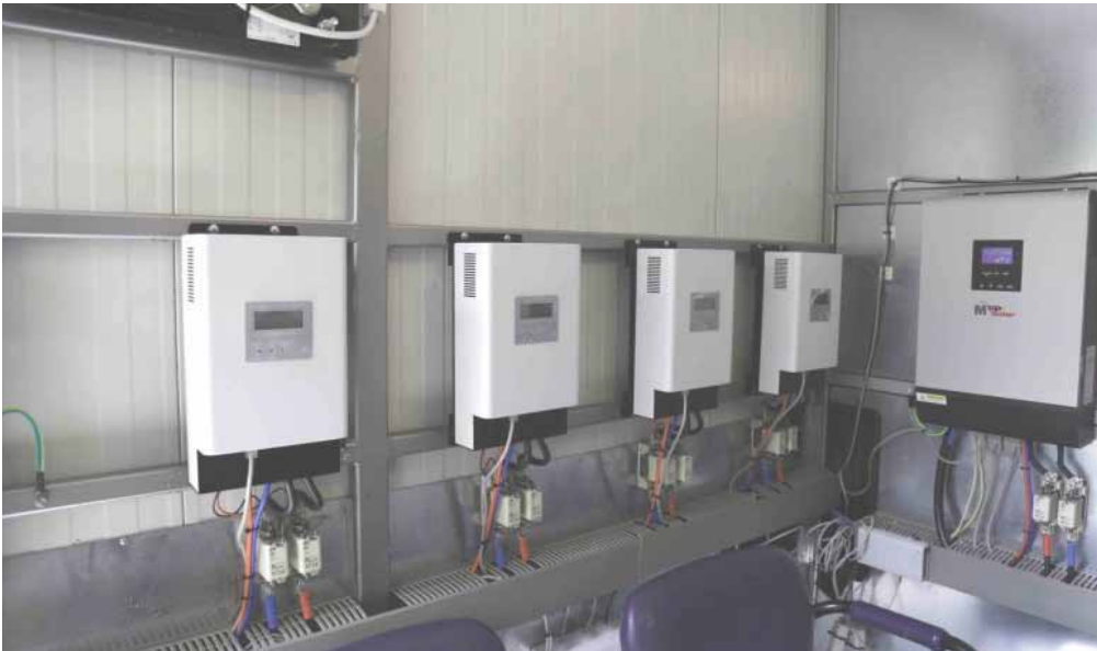
Compact Hybrid Power Plant at Power Development Board High School, Siddhirganj, Narayanganj, Electricity Company Bangladesh Limited.
