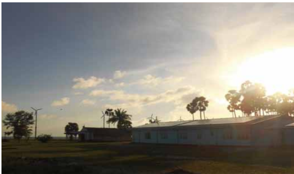
Solar PV array mounted on the roof of the power house: small-wind turbines in the background.
