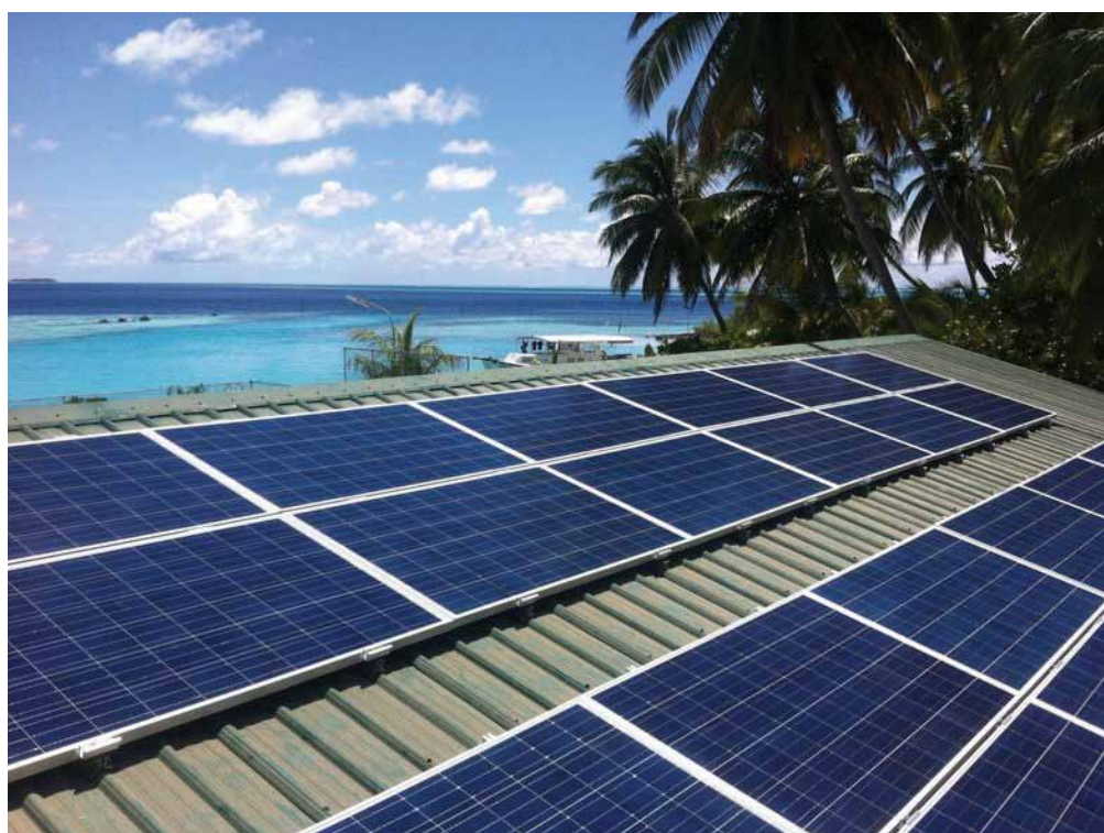
Photovoltaic Solar Power Plant on Rakeedhoo Island.
