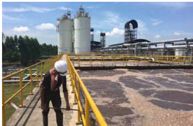
A worker taking out the pond scum at the E85 Wastewater Treatment Plant. Photo credit: E85.
