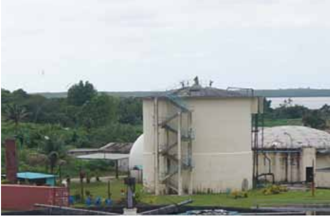
The Kinoya Sewage Treatment Plant with the new anaerobic digester and the biogas capture and flare system. Photo credit: Future Carbon Fund.
