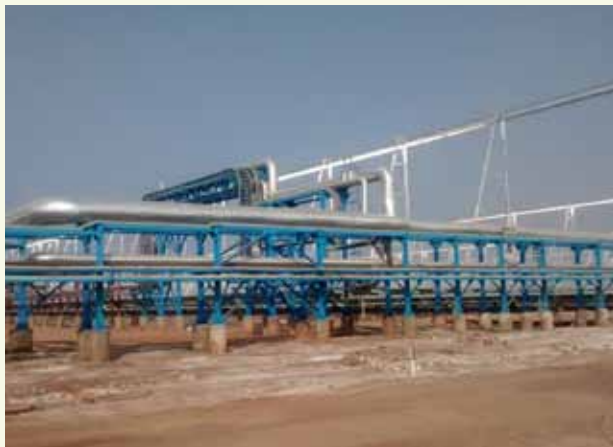
The 125-megawatt CSP Project at Dhursar village in Rajasthan. Photo credit: Future Carbon Fund.
