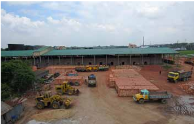
The Kapita Auto-Bricks plant. Photo credit: Industrial and Infrastructure Development Finance Company.
