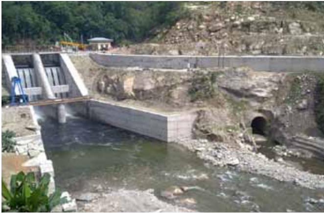
Diversion weir (downstream view) and connection channel of Dagachhu Hydropower Plant. Photo credit: Dagachhu Hydropower Corporation.
