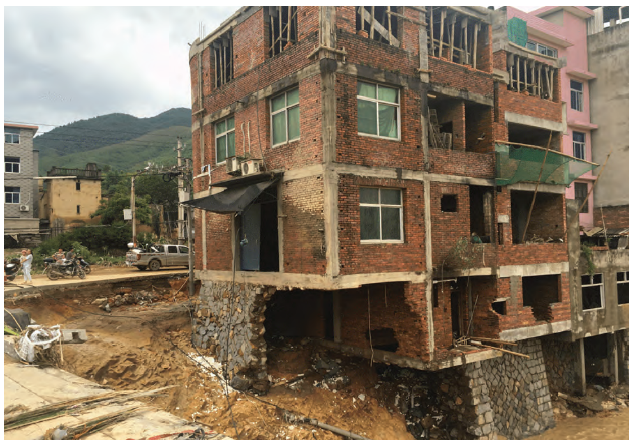
Devastation from flash floods in Minqing County. Collapsed roads and damaged buildings due to flash floods greeted residents of Minqing County, Fujian Province of the People's Republic of China in early July 2016 in the wake of super typhoon Nepartak (photo by the China Institute of Water Resources and Hydropower Research).
