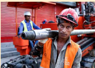
Trenchless technologies reduced disruption during the laying of water supply pipes in Dhaka.
