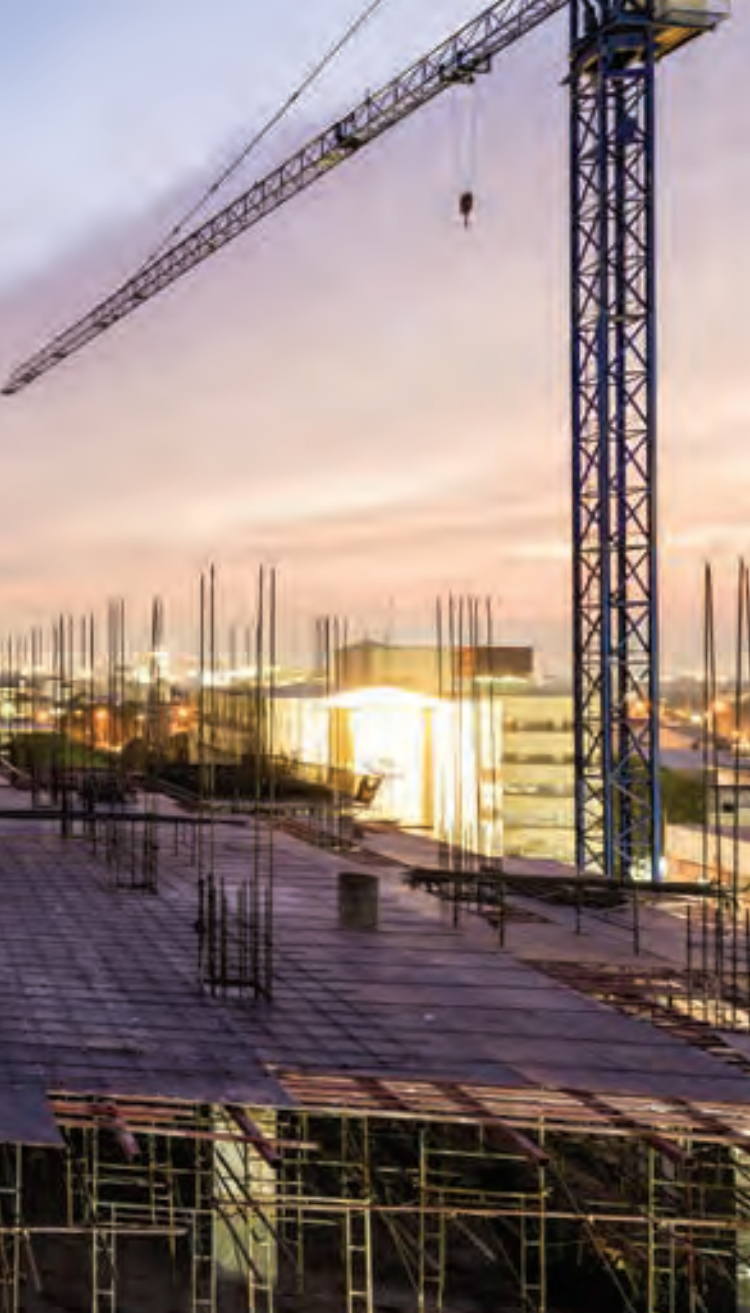
📷 ← The construction site of a new hospital in Chonburi, Thailand (photo from Shutterstock.com).
