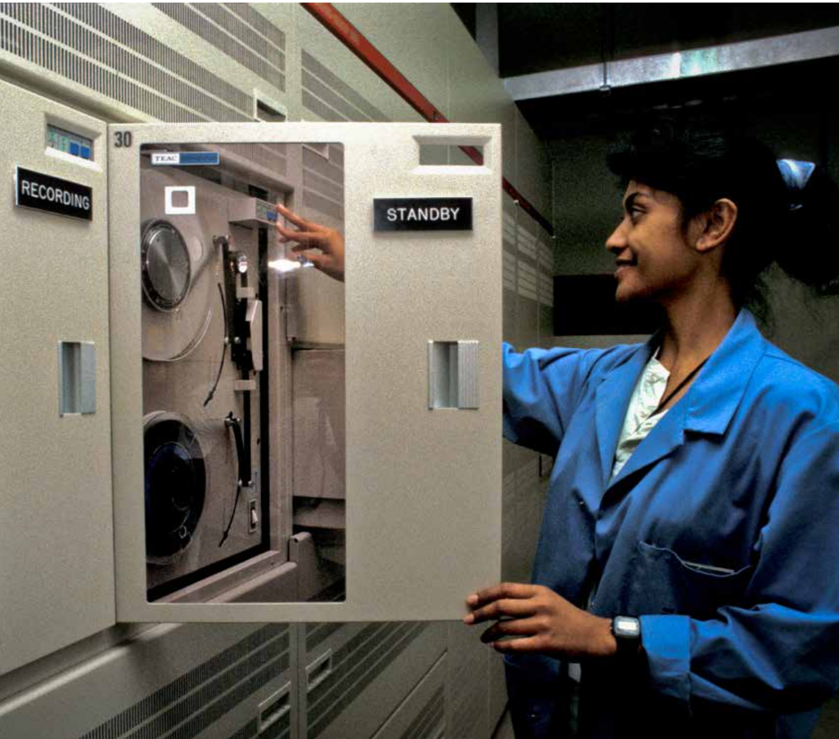
A woman checks on telecommunications equipment
