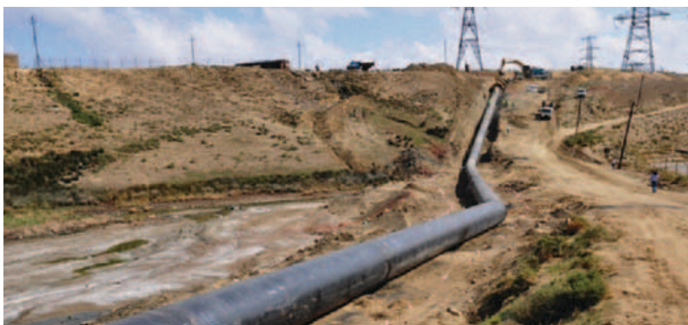
Expanding the water supply network. Azersu JSC is a full-service utility that designs, constructs, and maintains its own infrastructure, providing water supplies to over 1.3 million subscribers (photo by Azersu JSC).
