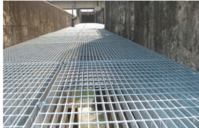
Fish ladder in the dam of the Babai Irrigation System. The dam has a fish ladder approximately 4 meters wide (photo by D.B. Swar).
