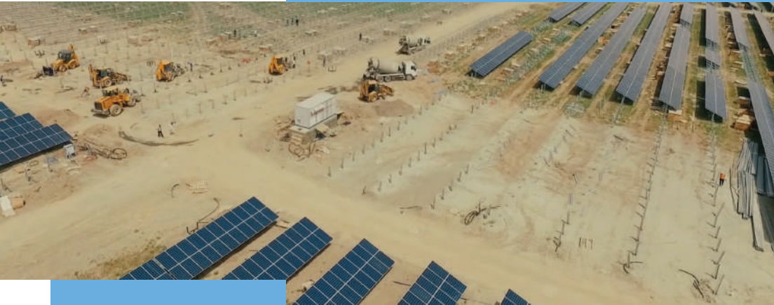
Solar panels being installed in Southern Kazakhstan (photo from Baikonyr Solar Limited Liability Company).
