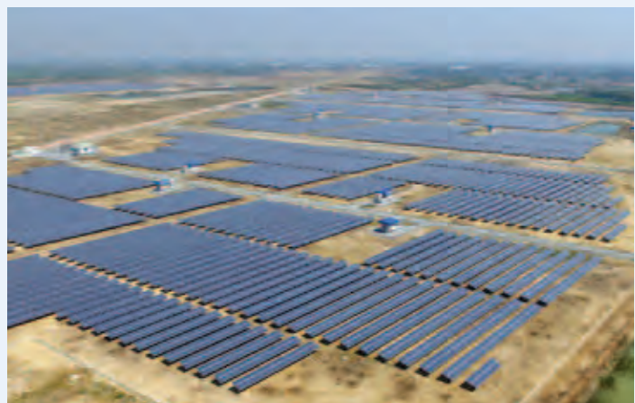
Thailand’s first certified green bond. ADB’s investment supported the construction and operation of 16 solar power plants with a total capacity of 98.5 megawatts (photo by B.Grimm Power Public Company Limited).
