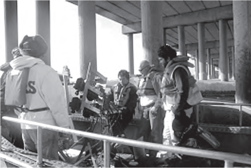
Inspection of continuous bridges at sea. West Nippon Company Limited efficiently investigates structures using digital and infrared cameras (photo by West Nippon Expressway Company Limited).
