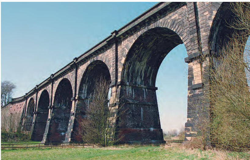
Sankey Viaduct of the Liverpool and Manchester Railway (United Kingdom). Completed in 1830, it is still in service (photo by Shunsuke Baba).
