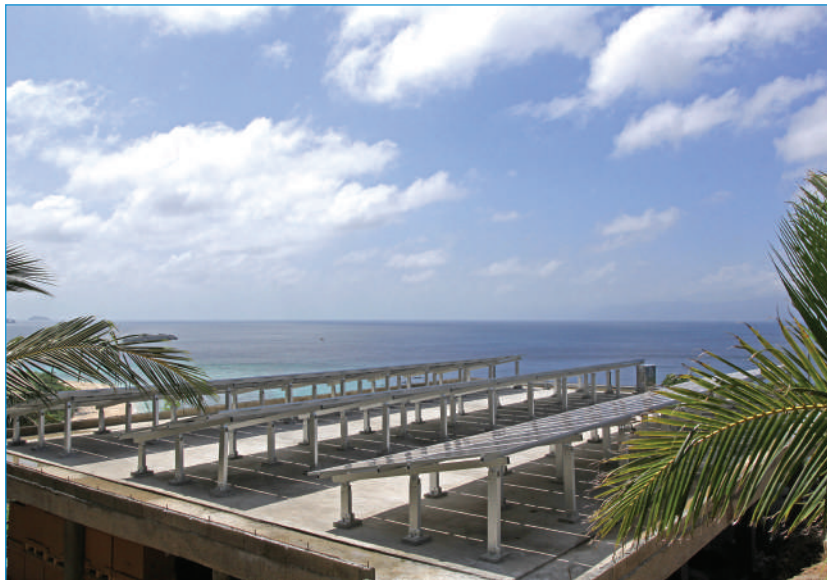
Powerhouse with Solar Photovoltaic Modules Installed at the Rooftop. The hybrid solar photovoltaic power plant is providing 24/7 electricity to the remote island of Cobrador in the Philippines (photo by Chrisanto George G. Quintana for Asian Development Bank).
