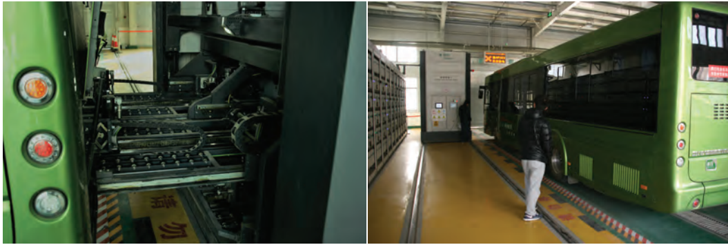
Battery swap station in Zhengzhou, People's Republic of China. Source: Asian Development Bank.
